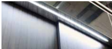
LED Lighting System embedded in the door frame
